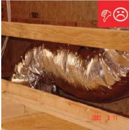
A. Duct is kinked in cavity.
