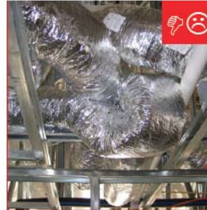
B. Ducts crammed into cavity, kinked and sharply bent.
