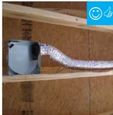
Fan housing was oriented in the correct direction to allow proper exhaust duct installation.
