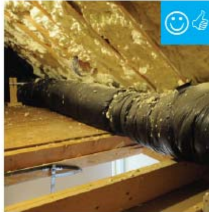
Duct is run straight and supported properly.
