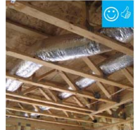
Ducts are run straight and supported properly.
