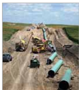
Kinder Morgan natural gas pipeline in western Nebraska
