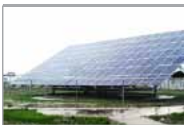
Solar array at Norfolk Operations Center
