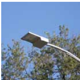
LED (Light Emitting Diode) street lights installed by OPPD from 45th to 46th on Woolworth Street in Omaha
