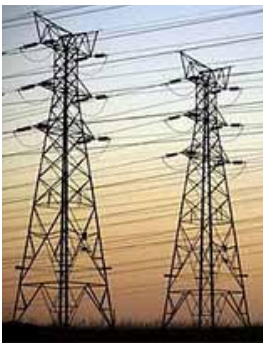
Western Nebraska transmission line.
