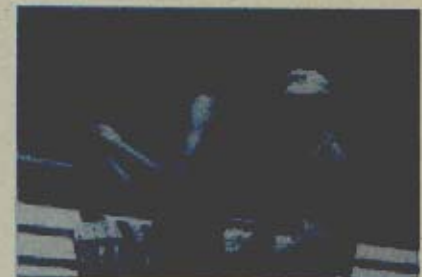
Two students caulk around window frames to eliminate air infiltration in one Auburn home.
