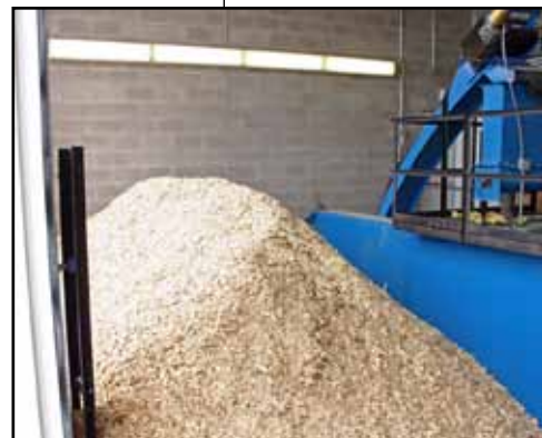
Chadron State College's woodchip fired boiler helps heat 20 campus buildings saving the college $360,000 each year.
